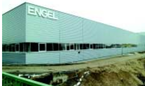
... have meanwhile been reclad, Once the interior had been cleared and refurbished ...
