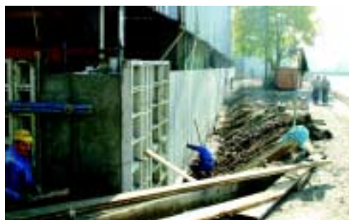
One of the walls of the machining shop had to be rebuilt and the walls ...
